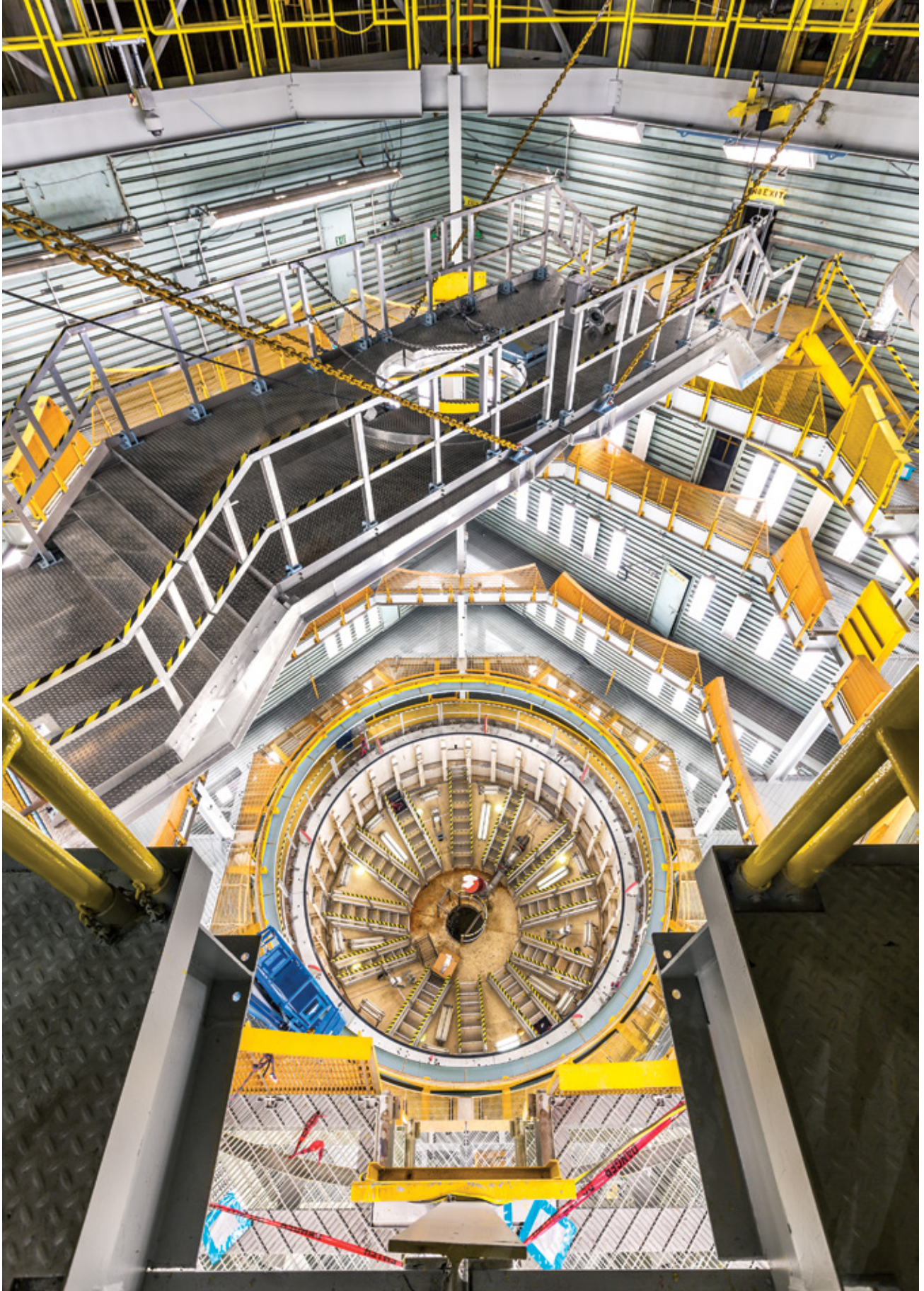
IN A HYDROSTATIC TEST CELL at Michoud, engineers pump water into the liquid-oxygen tank to check for leaks. In the fully assembled rocket, the oxygen tank will sit above a much larger liquid-hydrogen tank, the two separated by an “intertank” section.
