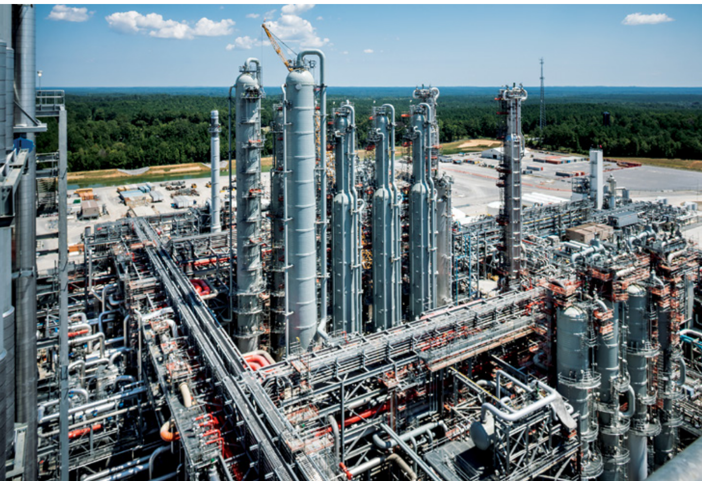
CAPTURING Kemper's CO 2 and other pollution requires the extensive labyrinth of ducts and towers shown above. The tall gasifiers that create the emissions are at the extreme left; power-producing turbines are out of view, to the right.
