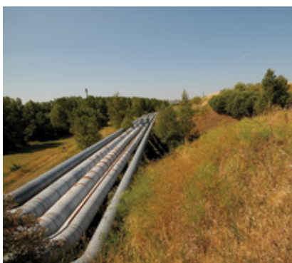
PIPES in Kalundborg, Denmark, carry waste steam from the DONG Energy power plant to companies that use it for manufacturing.
