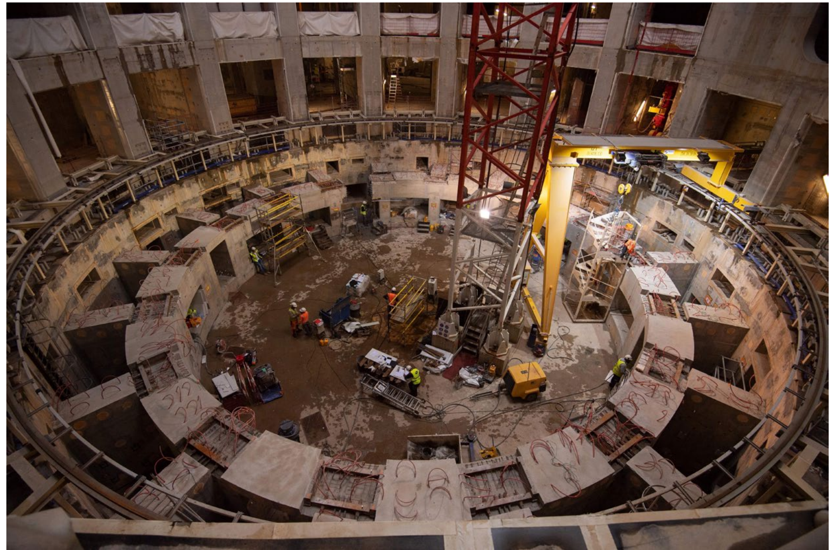
Employees work at the site where the tokamak confinement device will be installed.
