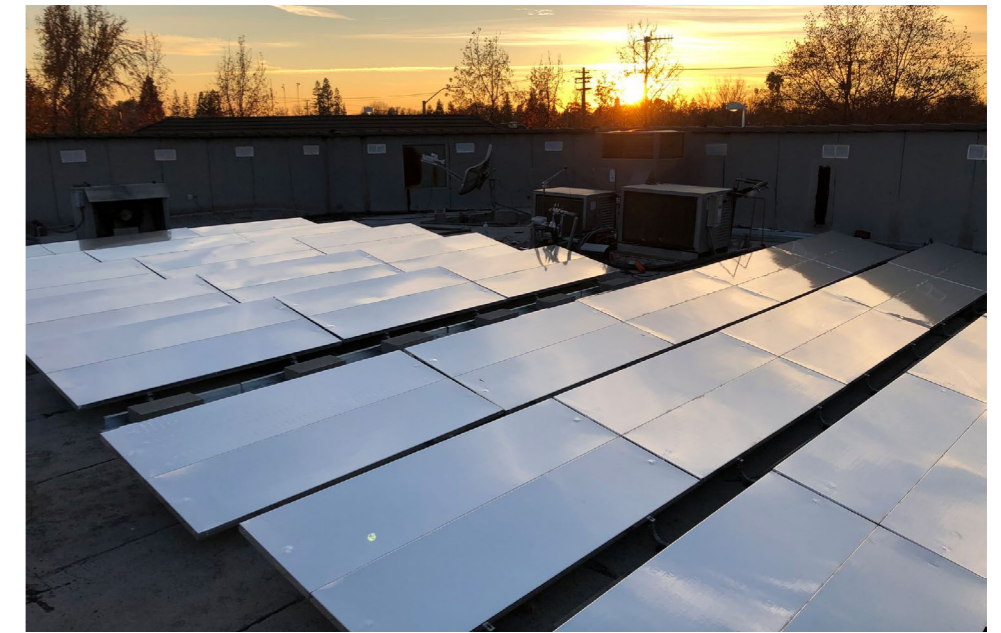
Supercool panels on the roof of a shop in Sacramento, Calif.
