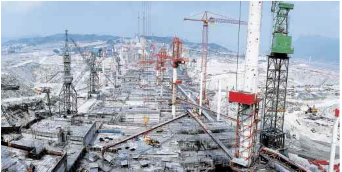
CONCRETE DELIVERY: Transporting concrete from the mixing plants to the dam requires a complex and extensive system of about five miles of fast conveyors ( above ). This equipment is raised by tower cranes as work progresses and the dam grows continuously taller.
